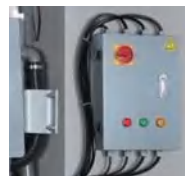
Total power source control dust collection box fault indicator
