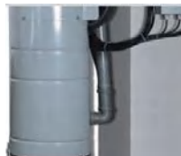
With automatic cleaning system of the filter, the filter effect of imported plastic film is better
