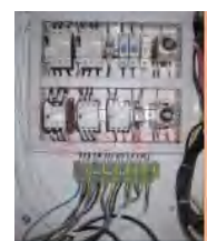
Schneider Circuit Breakers Schneider contactor Schneider thermal protector
