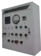
Automatic Control Box
